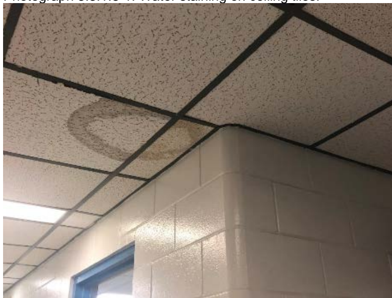
Photograph 3.3.1.8-1: Water staining on ceiling tiles.
