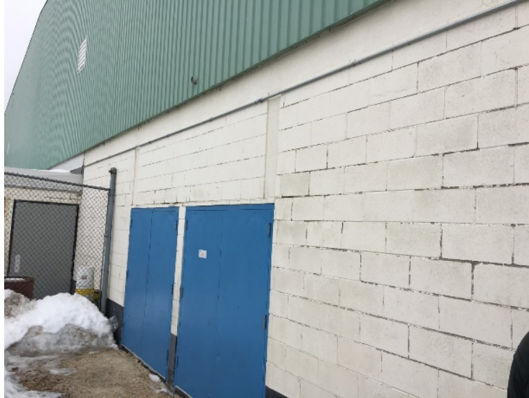
Photograph 5.2.1.3-3: Mortar joint deterioration of exterior concrete block walls.
