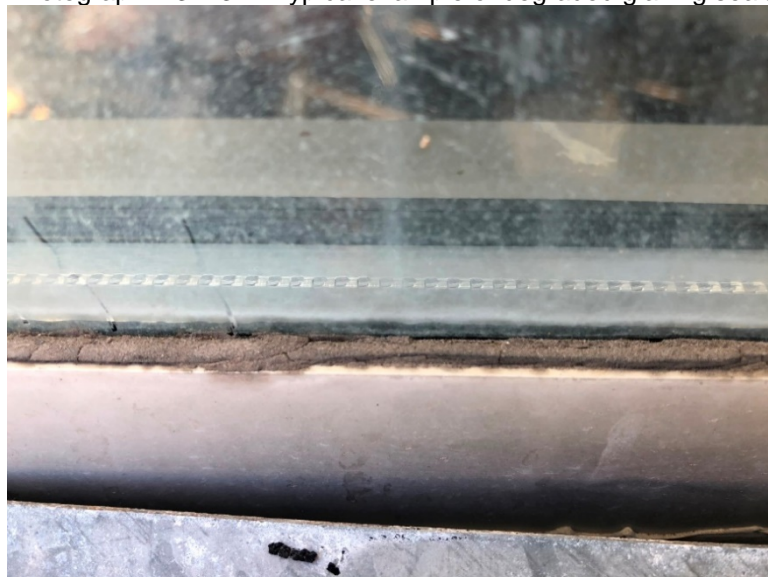
Photograph 4.3.2.3-3: Typical example of degraded glazing sealant and mildew growth at head and upper portion of the jambs.
