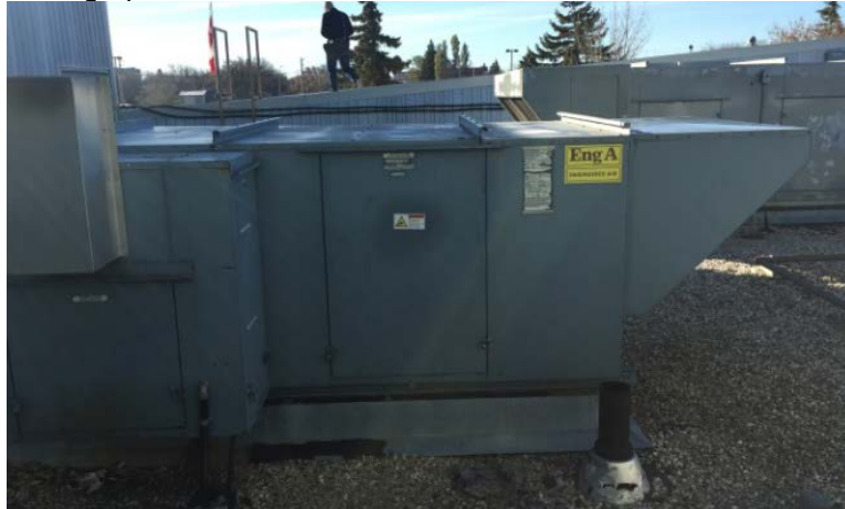
Photograph 2.5.3.3-1: AHU-3 Boiler Room Unit
