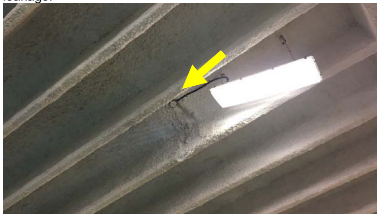
Photograph 4.2.4.2-1: Partial view of roof framing over pool showing evidence of past leakage.
