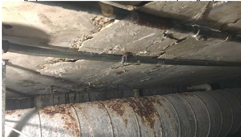
Photograph 4.2.2.1-1: Soffit delamination and spalling at pool tank drain.
