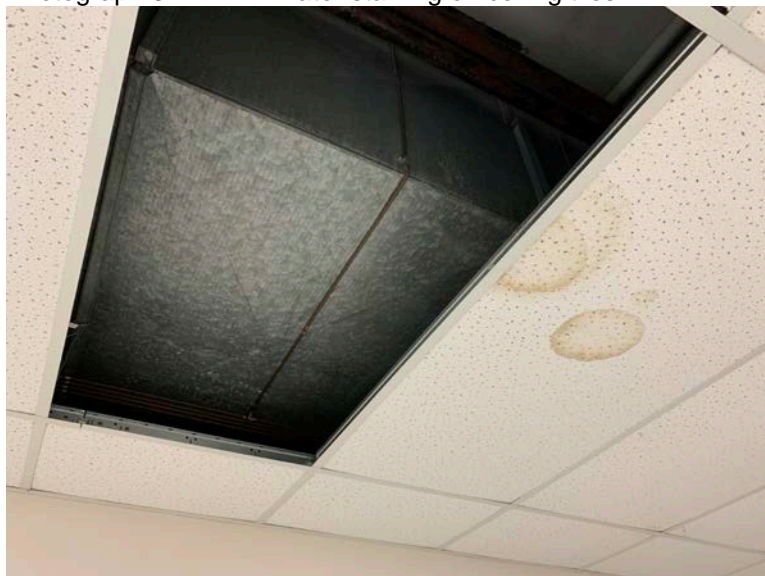
Photograph 3.2.1.2-1: Water staining on ceiling tiles.
