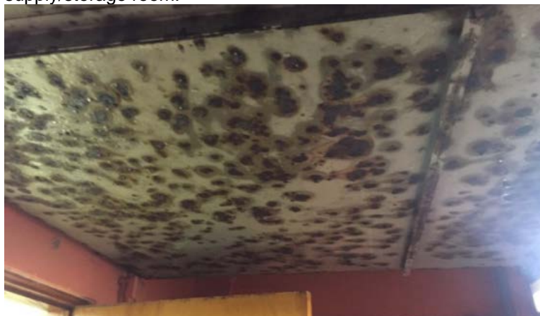
Photograph 4.4.1.1-3: Discoloured, corroded and pitted ductwork exposed in pool supply/storage room.
