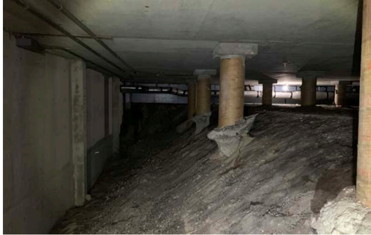
Photograph 3.2.1.1-2: Unfinished crawlspace floor show exposed soil.
