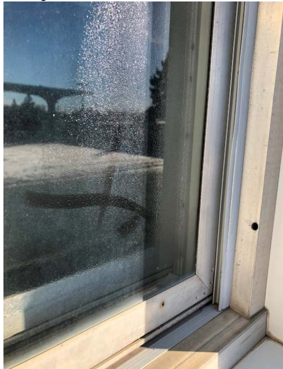
Photograph 4.3.2.2-2: Typical example of condensation accumulation on interior surface of the glass.
