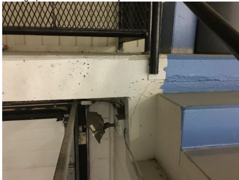
Photograph 5.2.1.5-1: Crack at joint between concrete bleachers and landing.
