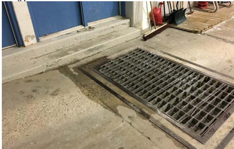
Photograph 5.2.1.4-1: Surface deterioration around snow melt pit. Concrete deterioration along joint and door sill.
