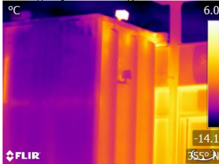
Photograph 4.3.1.3-2: View of thermal bridging at top of vertical concrete bands and along column supporting the entrance canopy, between the entrance and the open air above.
