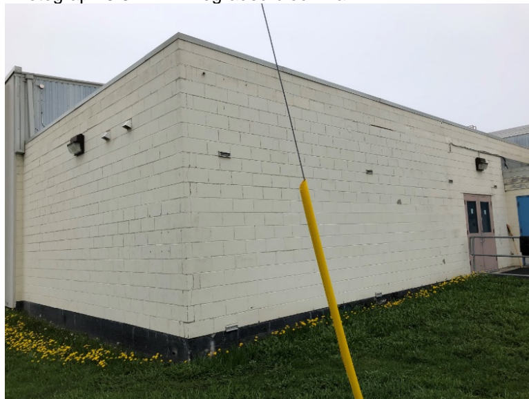
Photograph 3.3.1.4-1: Degraded block wall.
