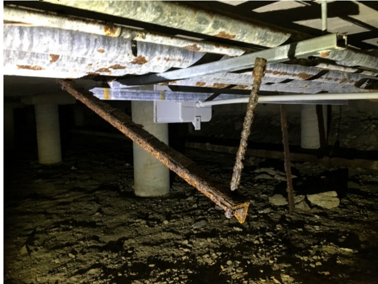
Photograph 5.2.1.1-3: Corrosion of conduits and hangers.
