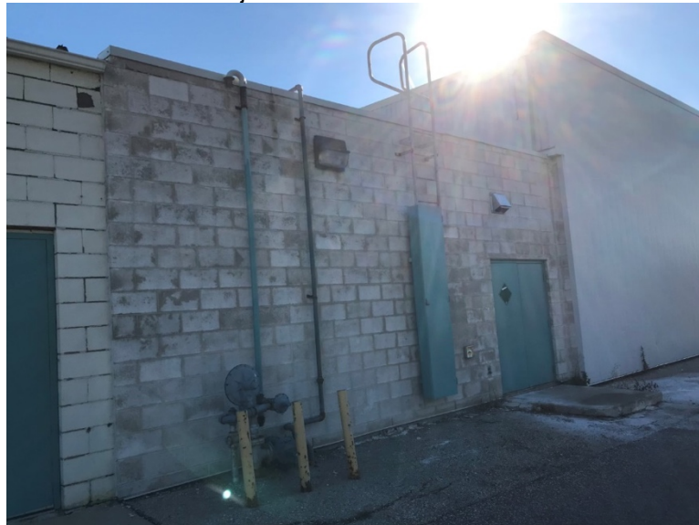
Photograph 4.3.1.3-5: Moisture stains at the existing masonry face block with localized block unit and mortar joint deterioration outside the women's locker/washroom.
