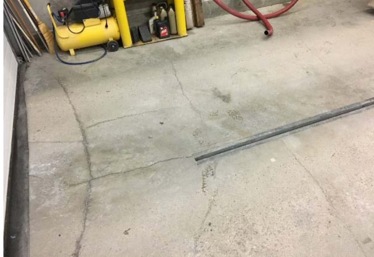
Photograph 5.2.1.4-2: Cracking in Zamboni storage room slab.
