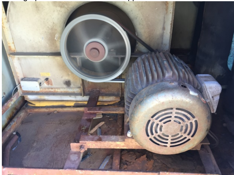
Photograph 4.4.1.1-1: Corroded supports for fan motor
