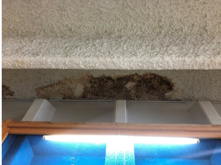
Photograph 3.3.1.6-2: Water staining on ceiling along the east wall.
