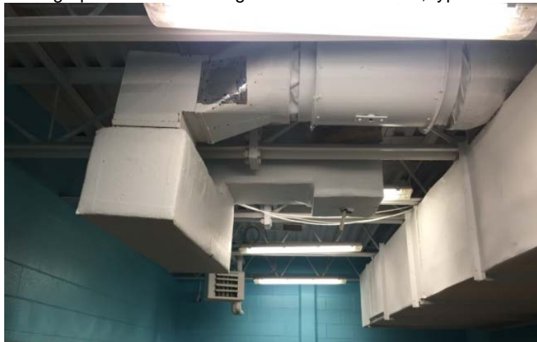
Photograph 2.5.3.4-1: Change Room Exhaust Fan, typical for each change room.
