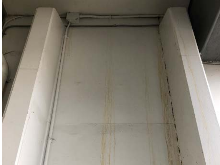
Photograph 3.3.1.5-1: Water staining at main entrance.
