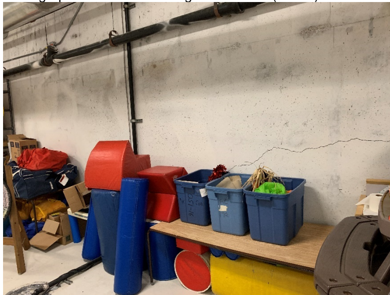
Photograph 3.2.1.3-2: Cracking in north wall (centre).
