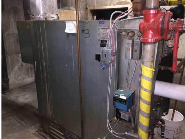
Photograph 2.5.2-1: Domestic Water Boiler
