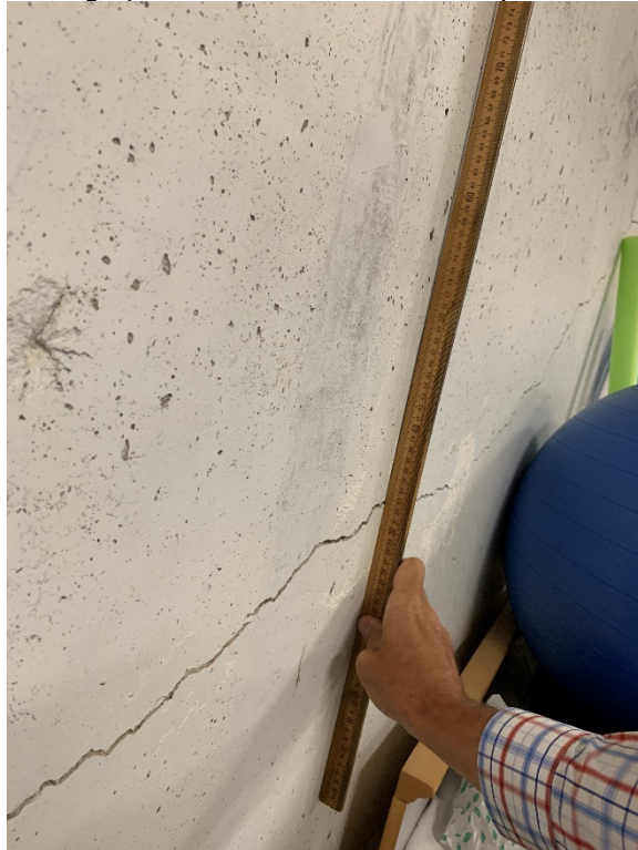
Photograph 3.2.1.3-4: Evidence of displacement in wall.
