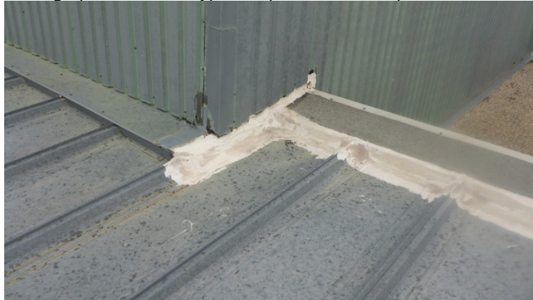
Photograph 5.3.2.3-2: Typical repair on a metal panel.
