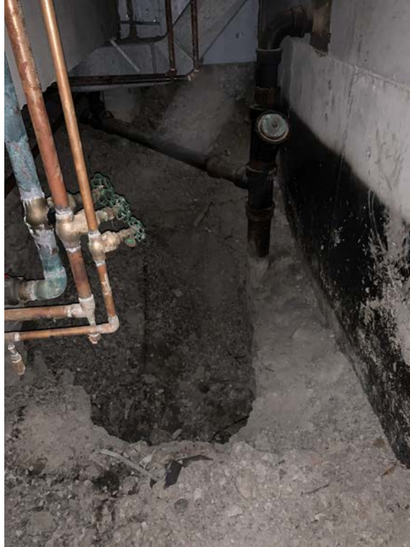
Photograph 3.2.1.3-4: Evidence of displacement in wall.
