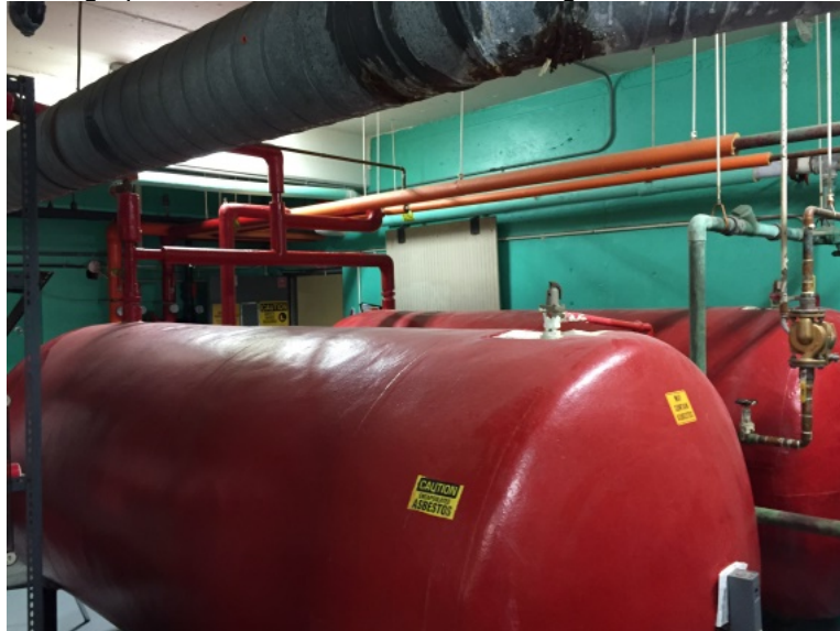
Photograph 2.5.2-2: Domestic Water Storage Tanks
