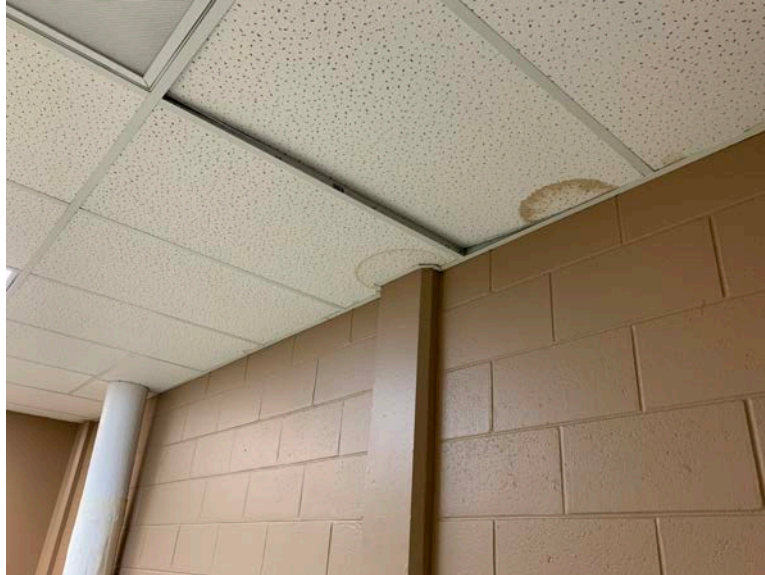
Photograph 3.2.2.1-2: Evidence of leakage along the transition from the low roof over the hall to the stairwell.
