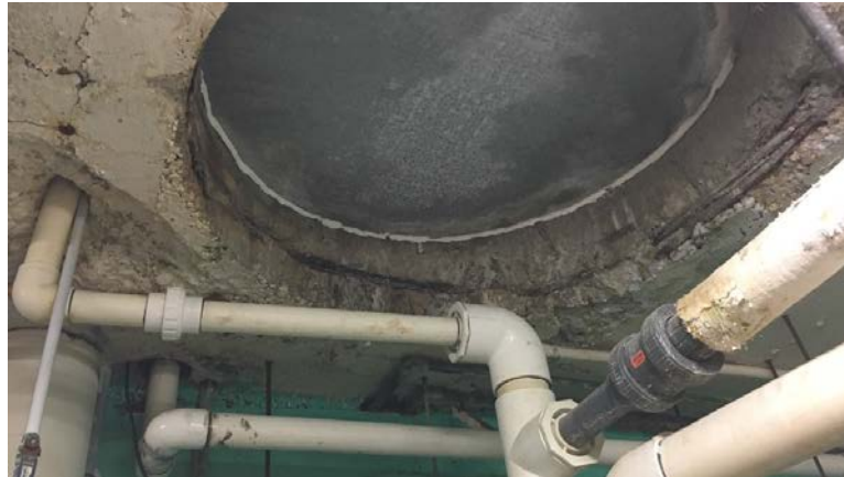
Photograph 4.2.2.1-3: Concrete repairs and deterioration around opening in the main floor slab.
