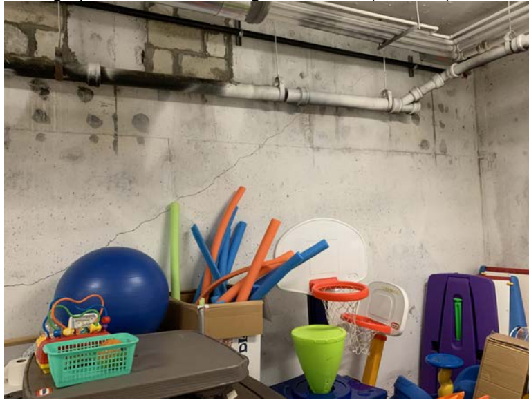
Photograph 3.2.1.3-1: Cracking in north wall (east end)
