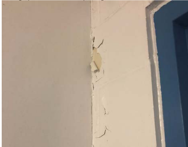
Photograph 3.3.1.4-6: Paint peeling from concrete block.
