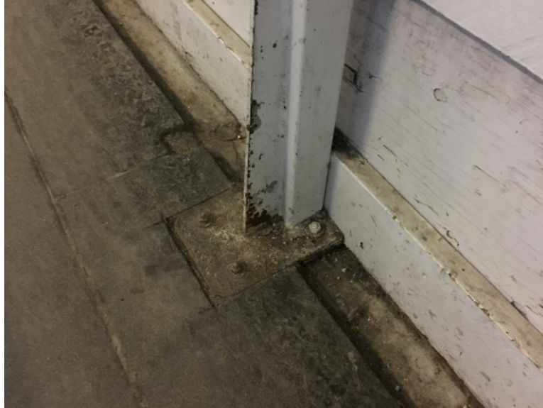
Photograph 5.2.1.7-1: Corrosion on dasher board framing.
