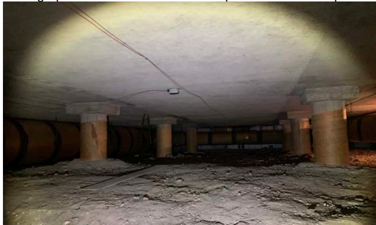
Photograph 3.2.1.1-1: Unfinished crawlspace floor show exposed soil.
