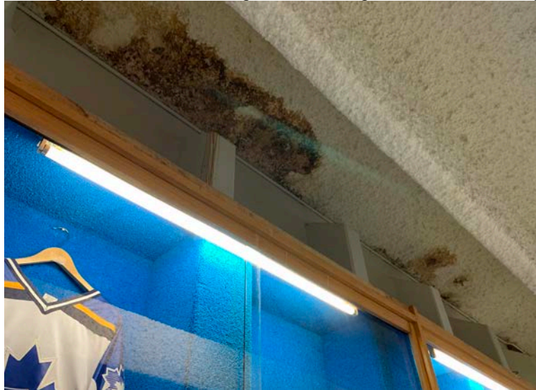
Photograph 3.2.2.2-1: Leakage visible along transition from lobby roof to auditorium roof.
