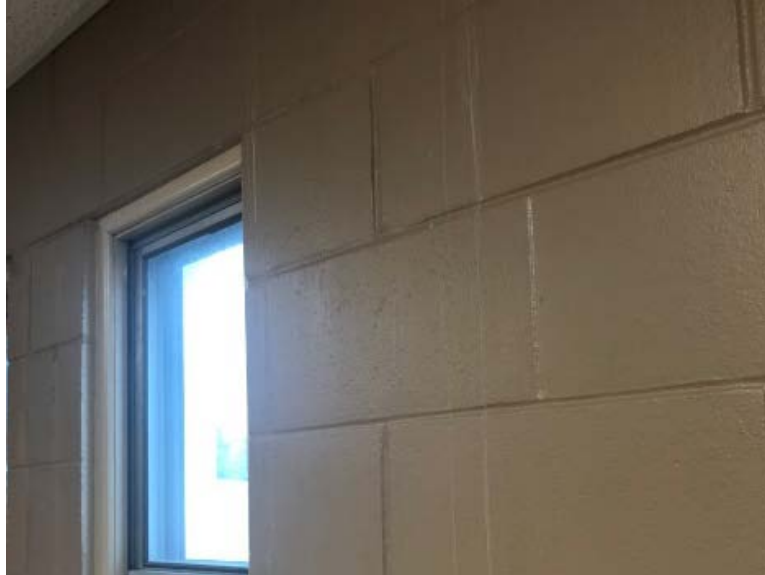
Photograph 3.3.1.13-1: Water staining on concrete block.
