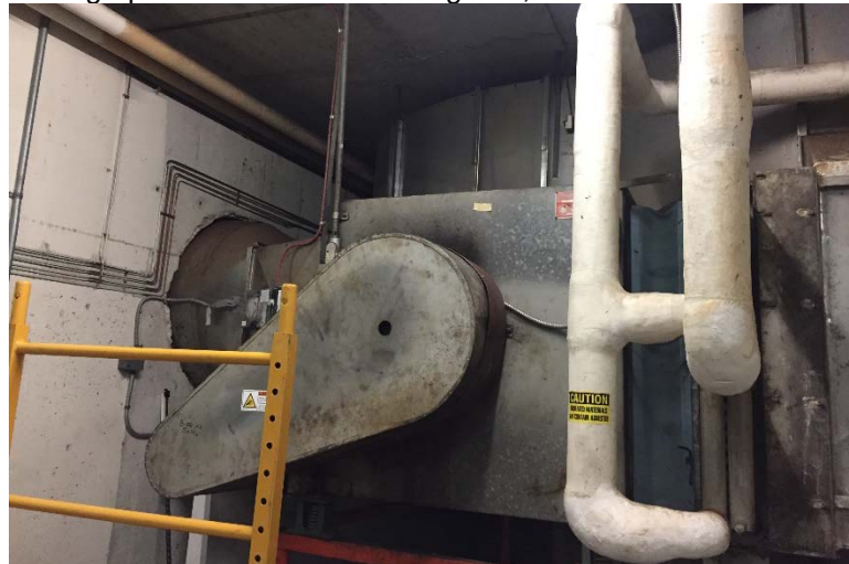
Photograph 2.4.4.1-1: Air Handling Unit, AHU-1
