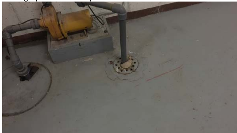
Photograph 4.2.1.4-1: Spall at floor slab.
