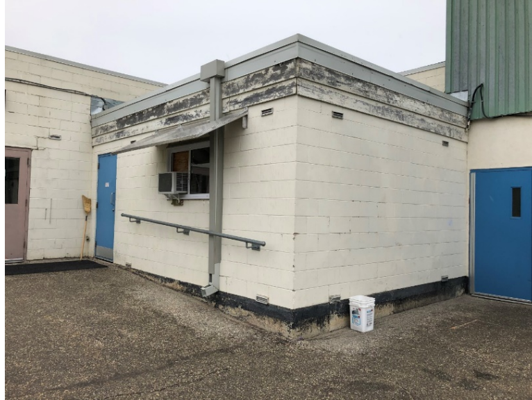
Photograph 3.3.1.4-4: Degraded block wall and weathered wood trim.
