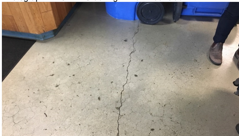
Photograph 4.2.3.2-1: Cracking in main floor slab.
