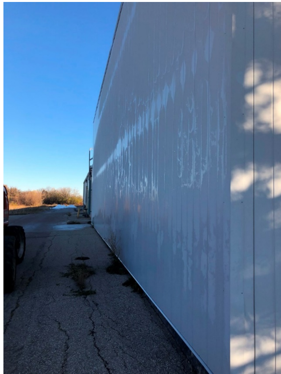
Photograph 4.3.1.3-3: Condensation observed at the existing metal cladding along the West elevation.
