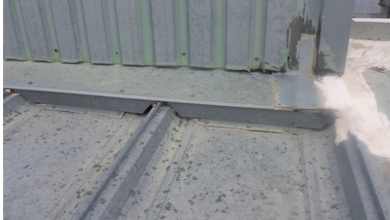
Photograph 4.3.3.3-2: Showing repair at roof wall interface.
