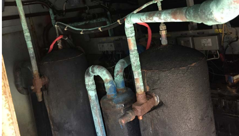
Photograph 4.4.1.1-2: Failed Compressors in AHU-2
